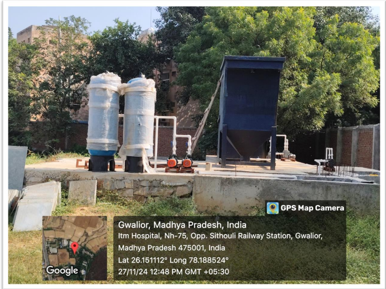
Photos of STP and ETP Installed
